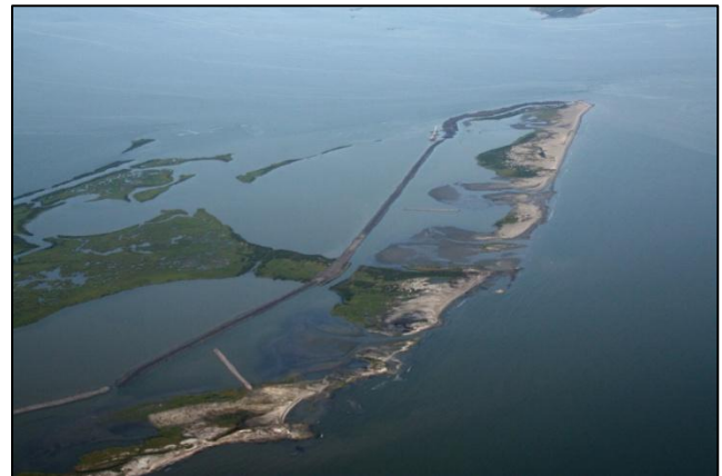
Aerial View of East Grand Terre during primary dike construction but prior to fill placement.
